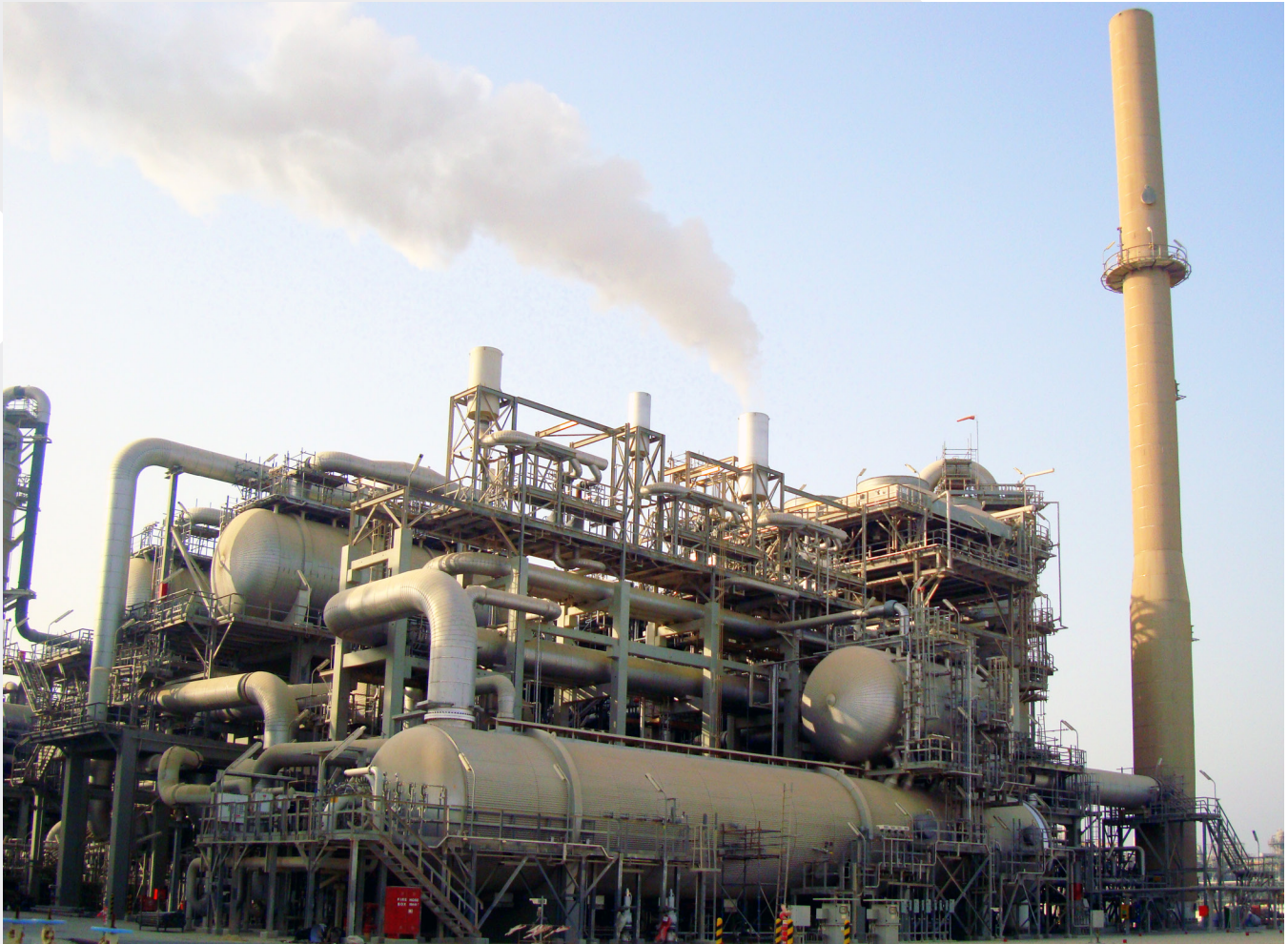
SRU Tail Gas Thermal Oxidizer with firetube style waste heat boiler.
