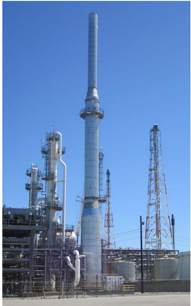
Vertical SRU Tail Gas Thermal Oxidizer
