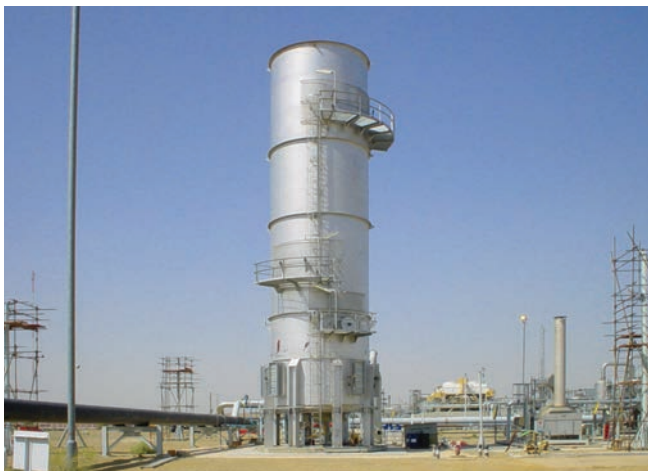
Vertical SRU Tail Gas Thermal Oxidizer
